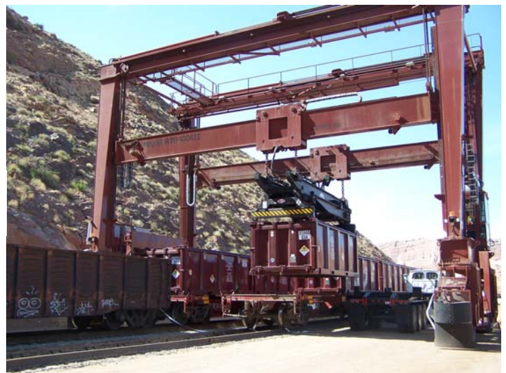
(Right) The gantry crane is loading a container of tailings onto a railcar.
