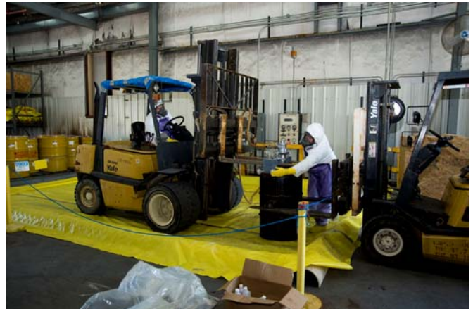
Workers performing the solidification of mineral oil for Alpha 5 at Y-12 facility.
