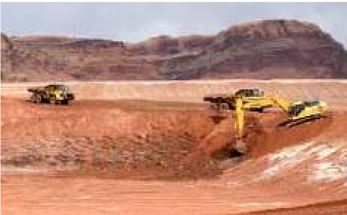
(Left) A track hoe excavates tailings from the pile into a dump truck that takes them to a drying bed where they are conditioned for disposal.
